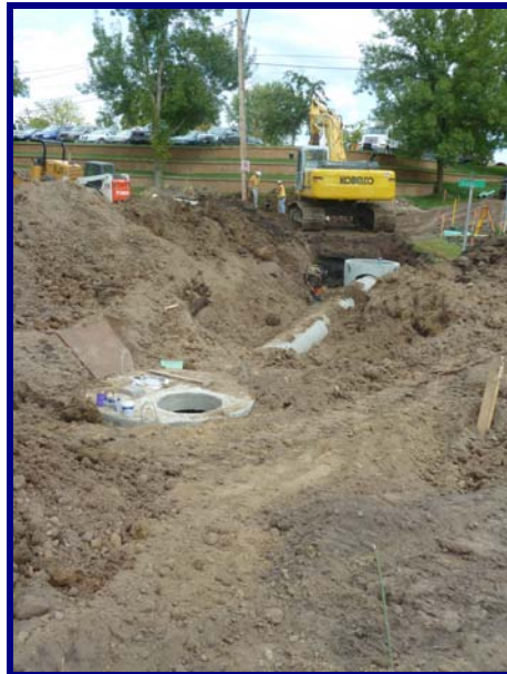
Installation of the stormwater separator—southeast corner of the Government Center parking lot
