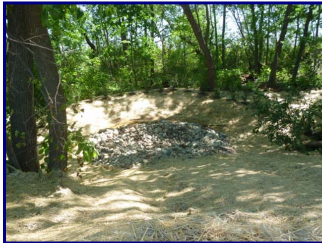
View looking down into the gully, towards Green Lake. Rocks were placed at the base of the gully to diminish bottom erosion; straw and netting were placed on the slope of the gully to encourage seed establishment.
